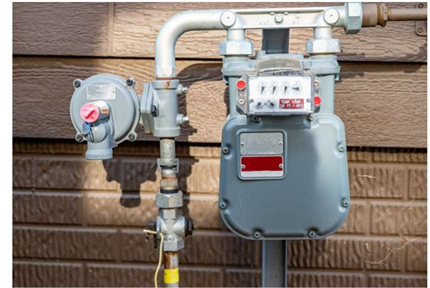
Gas regulator and meter
