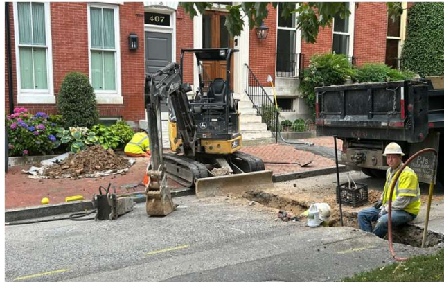
Gas service line
